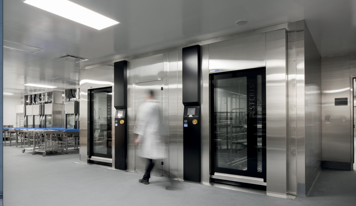
↑ Sterilisation room and equipment, view from unsterilized zone
